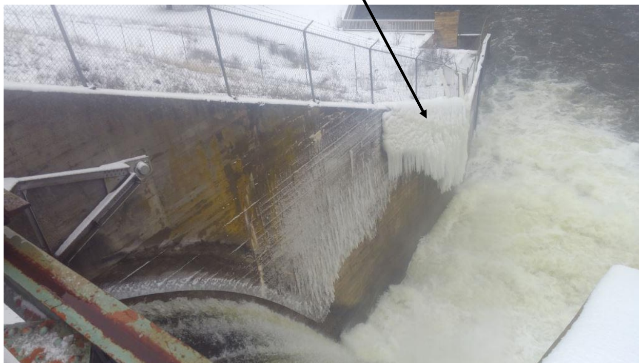
Edenville Dam, Tobacco River Spillway: View of Left Side Gate Oriented Downstream (22 December, 2017)
